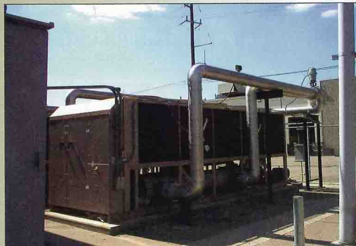
A slab-mounted air-cooled chiller supplies chilled water to interior air handling units, while a redundant chiller stands ready in the background.
