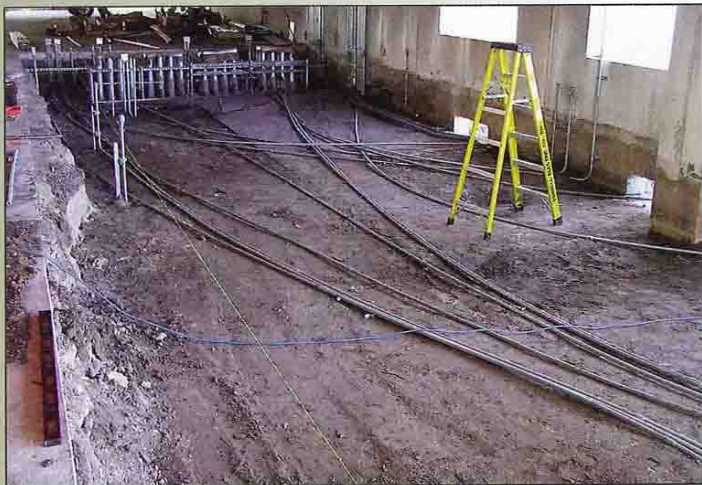
Compacted top-soil over a duct bank in preparation for electrical switchgear and a 12,000-gallon fuel tank to be housed inside an explosion-proof room.
