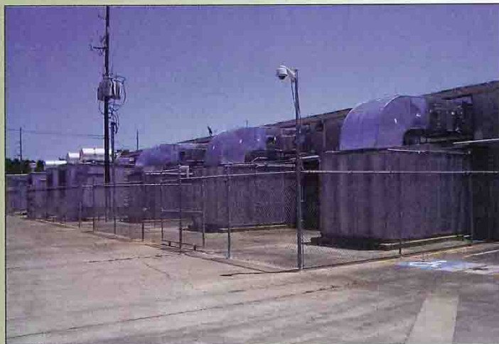
A fence and a video camera in plain sight deter unauthorized access to this arrangement of three generators in the background and three mechanical air handling units in the foreground.
