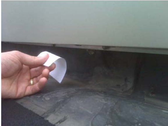
Figure 1. Air leakage bends paper at roof column exposure.
